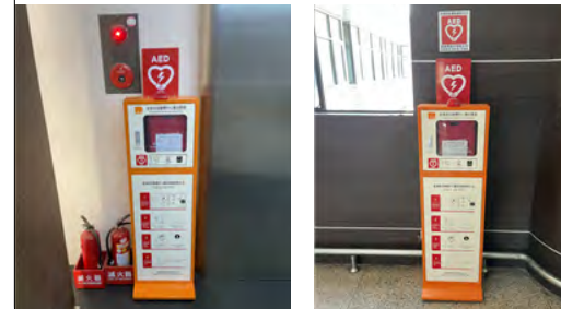
AED Devices Installed in the Taiwan Office and Manufacturing Facilities
