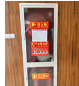
Fire Protection Facilities at Jiangsu Wieson
